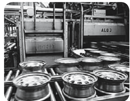
Aluminium age-hardening furnace with air/gas ratio controls for air deficiency cut-out
