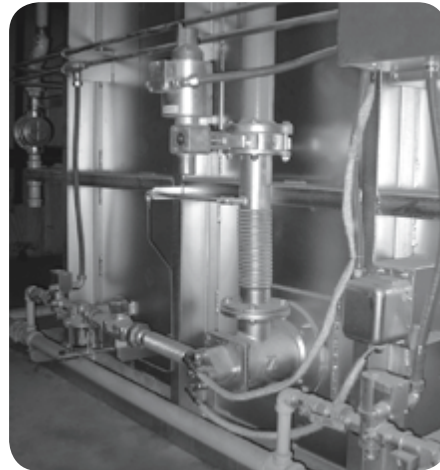
Chamber furnace in the refractory industry heated with excess air burners BIC 140LB.
