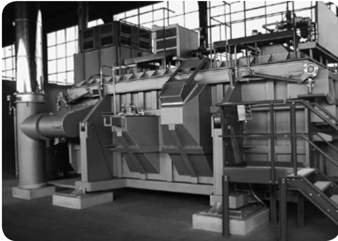
Aluminium industry: smelting furnace
